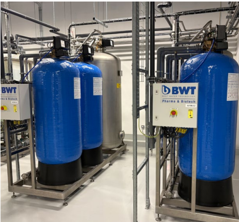
↑ Pre-treatment, UV filters, water softening and carbon filtration skids
