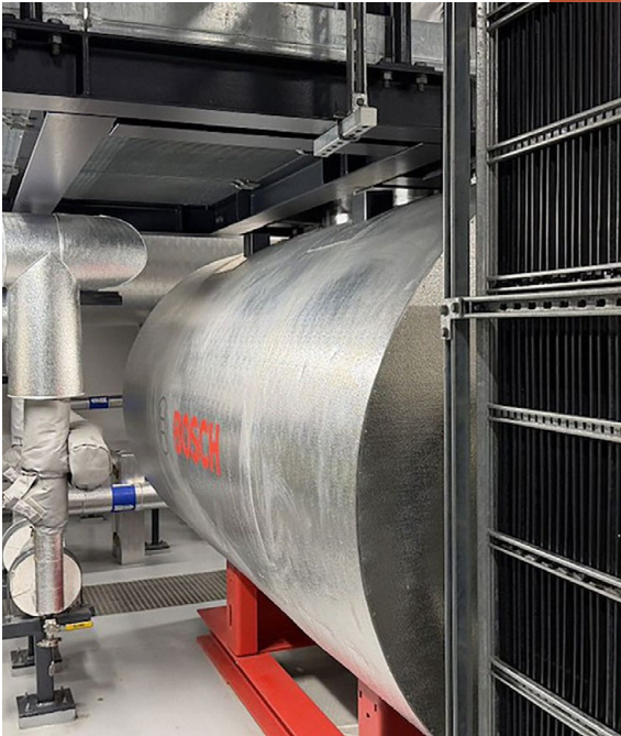
← Electric boilers in Milky Way
