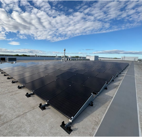
Roof solar panels ↓
