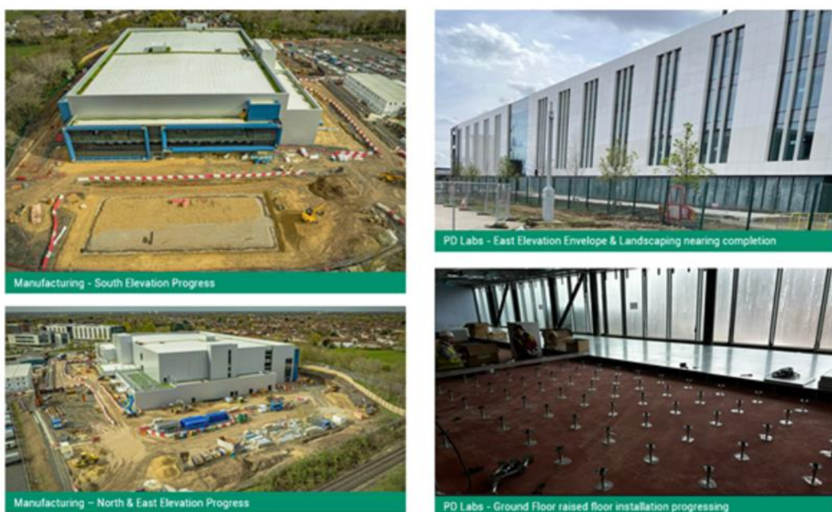
Fig 2. Single-use cell culture facility expansion at FDB's Billingham, UK site, progress as of October 2024.
